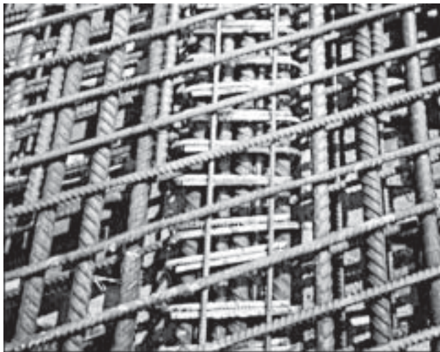
Fig 2 Congested reinforcement (should be avoided)
